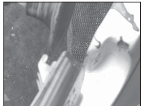
PHOTO 10 An angle grinder with a small disc is being used to touch up the tab.
